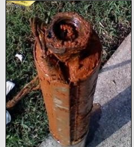
This pump was ruined within two years due to iron deposits.
